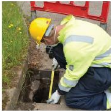
Clean gully of debris and measure for width, height and depth.
