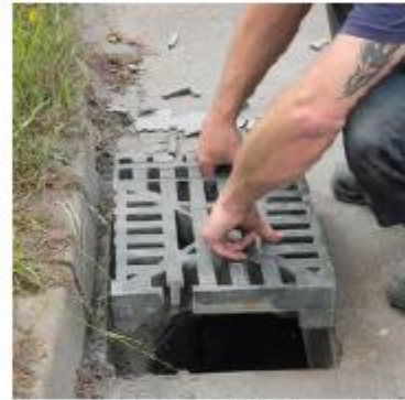
Drop grate into place and check for final fit - it should not rock or be proud of the roadway.
