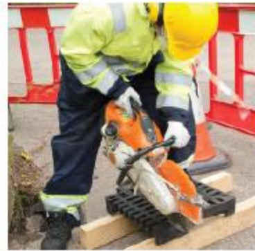
Using a power saw or angle grinder with a masonry disc cut grate to size.
